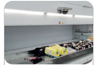
External Bay Lighting
